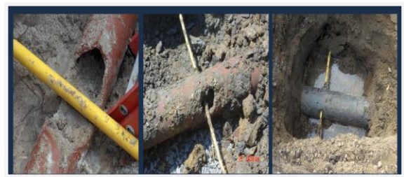
GAS LINES BORED THROUGH SEWER LINES (CROSS BORES)
